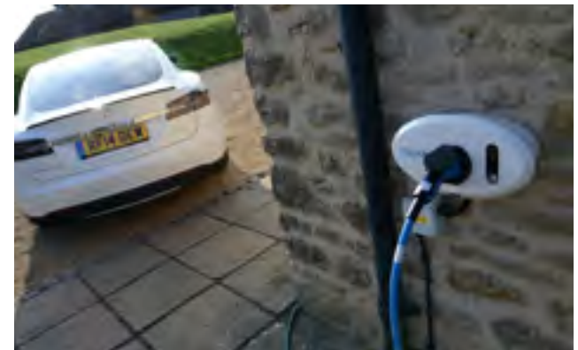
Figure 82: Example of off-street electric vehicle charging points.
